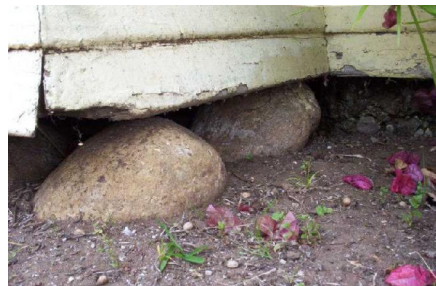
Figure 5. River rocks being used to support the foundation.
